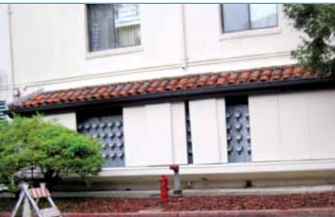
180 Smart Meters installed in US apartment complex
